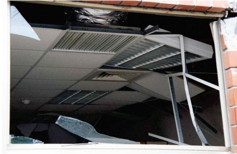
Figure C13.1-4 Damaged ceiling system.
