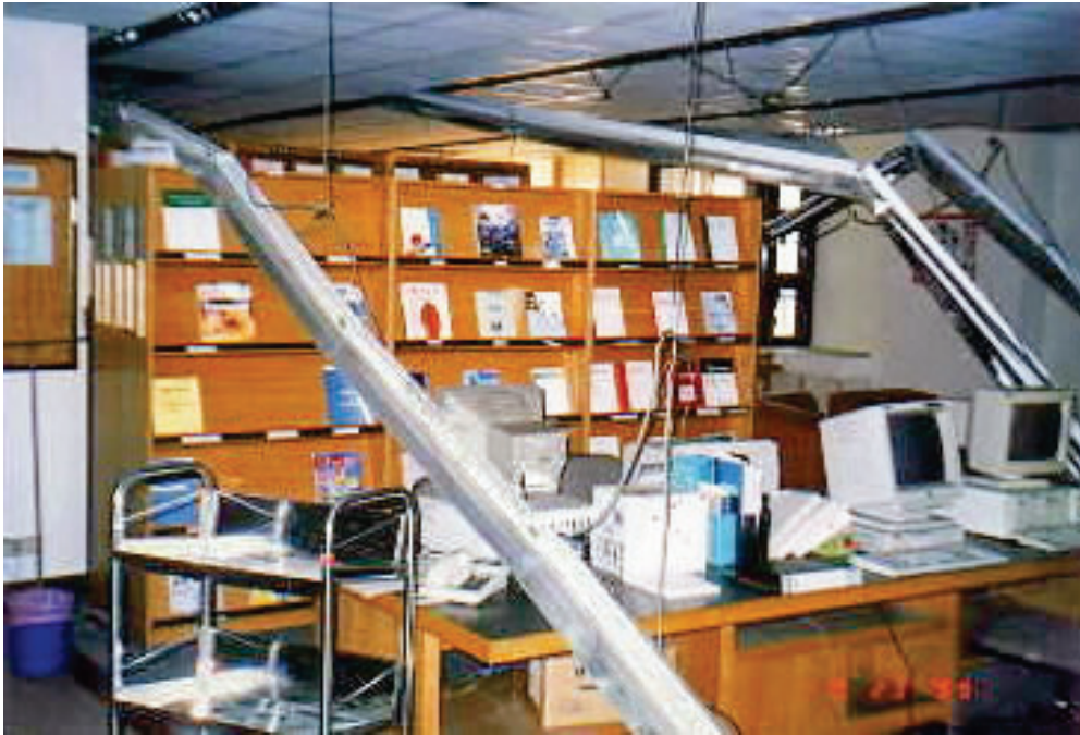
Figure C13.1-2 Collapsed light fixtures.
