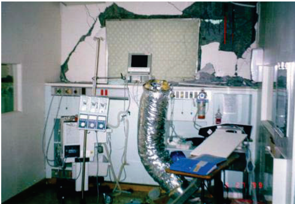
Figure C13.1-3 Collapsed duct and HVAC diffuser.
