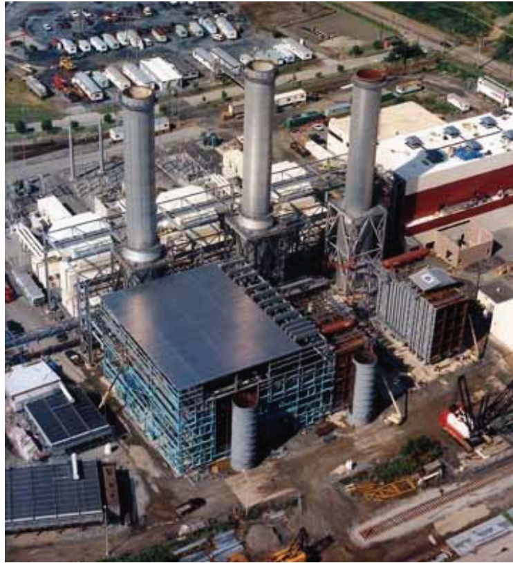
Figure C15.1-3 Heat recovery steam generators.
